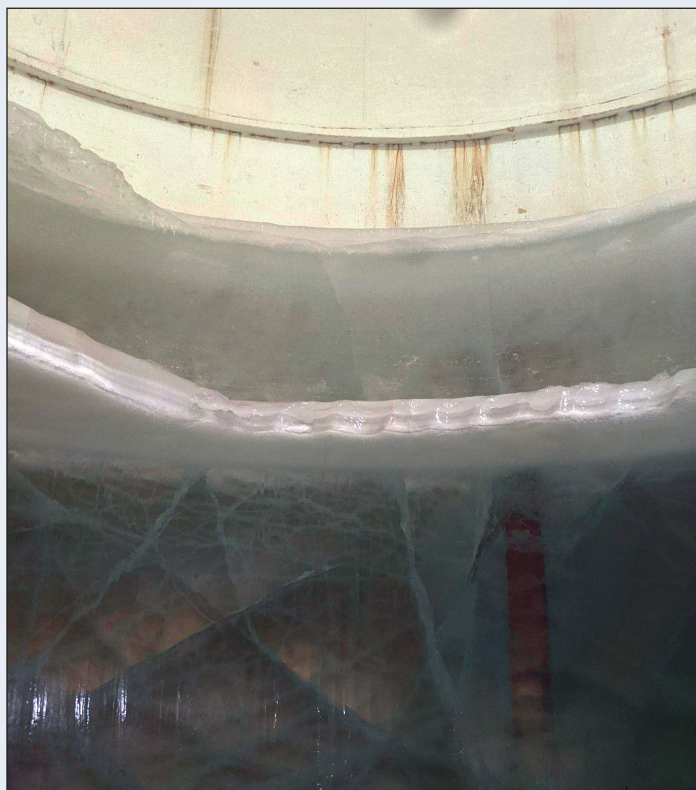
Ice build-up in tower.
